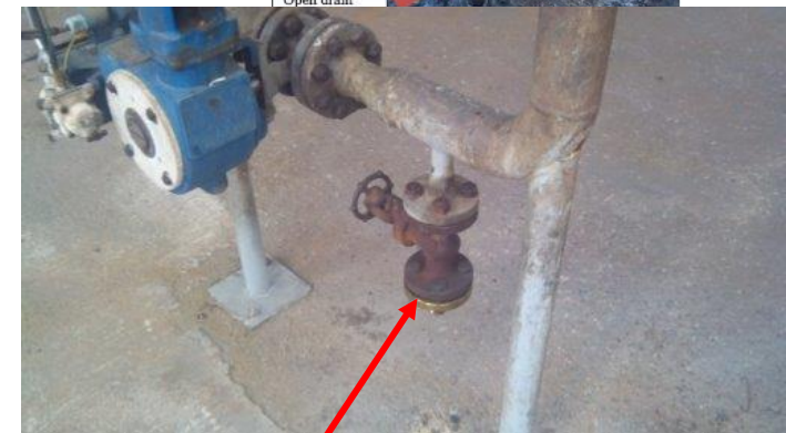
Manual valve open with no blind
